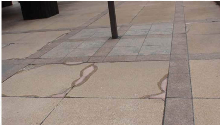
Existing Paver Distress
