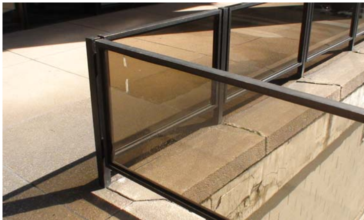
Existing Handrail Distress
