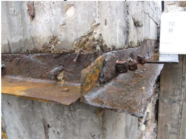
Existing Corroded Shelf Angles
