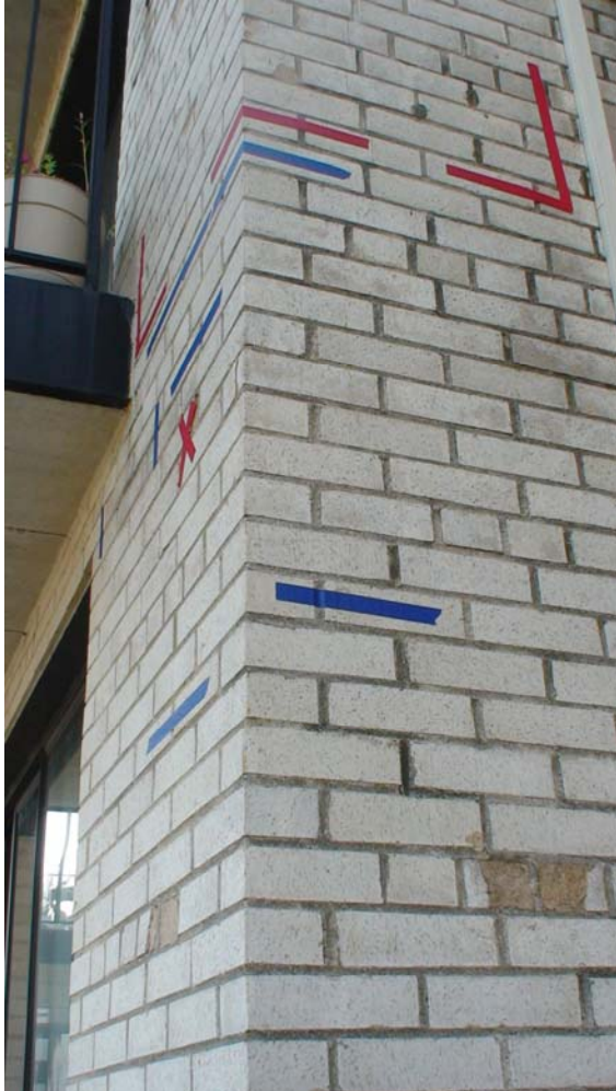
Existing Visible Distress for Prototype Wall Replacement
