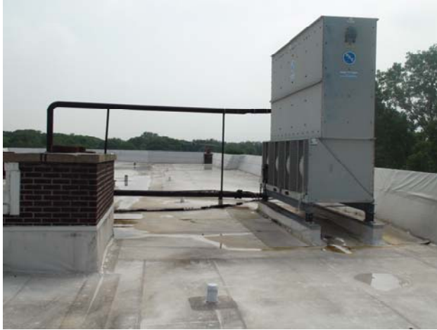
View of Existing Damaged Roof
